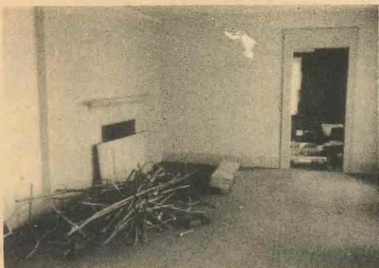
BEFORE: The Kiekhofer's faced cleanup and remodeling before they could move in. This fireplace wall is modern. It has been completely removed and an antique replacement installed.
