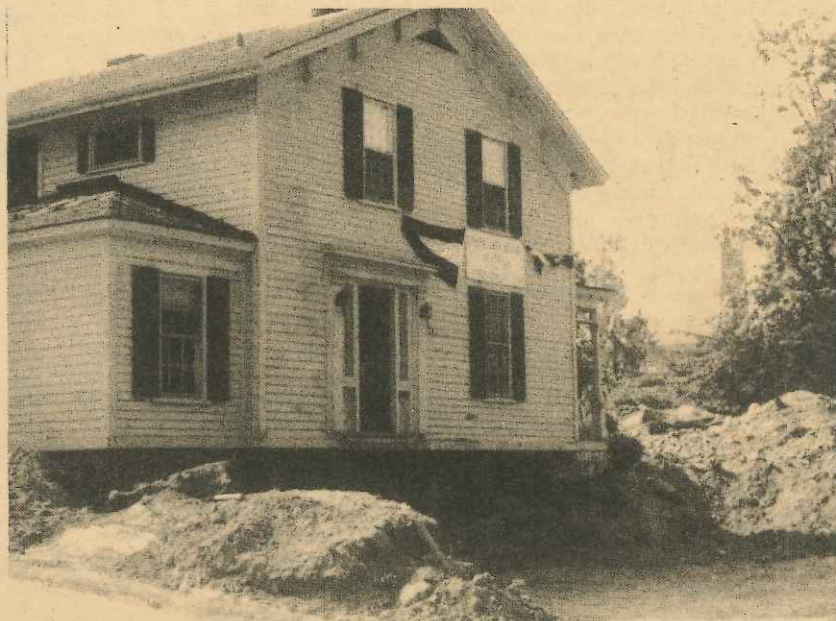
The foundation is removed from under the 124 year old Luther Clapp house and..
